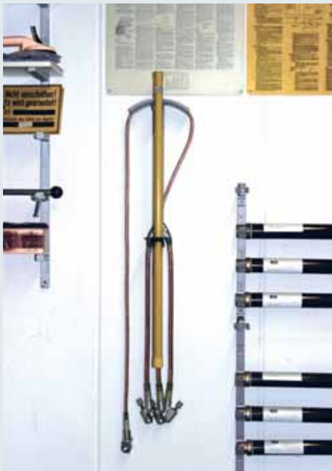
Storage device for earthing and short-circuiting devices and earthing rods.
