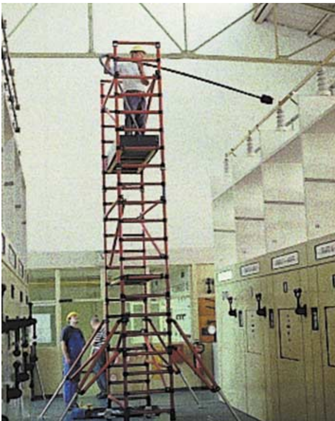
Figures 4 a and b: Cleaning of 30 kV rated switchgear from an insulated platform
