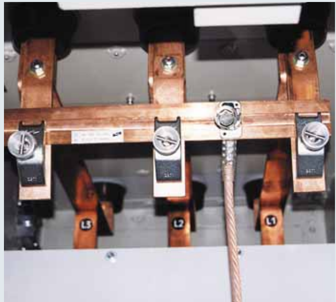
Short-circuiting bar with earthing cable in use at a switchgear.
