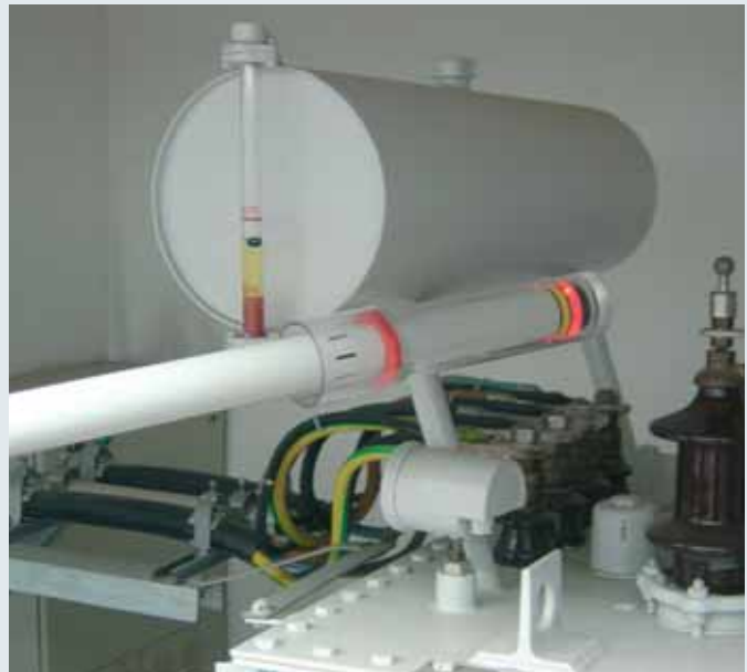
Distance voltage detector used for a switchgear.
